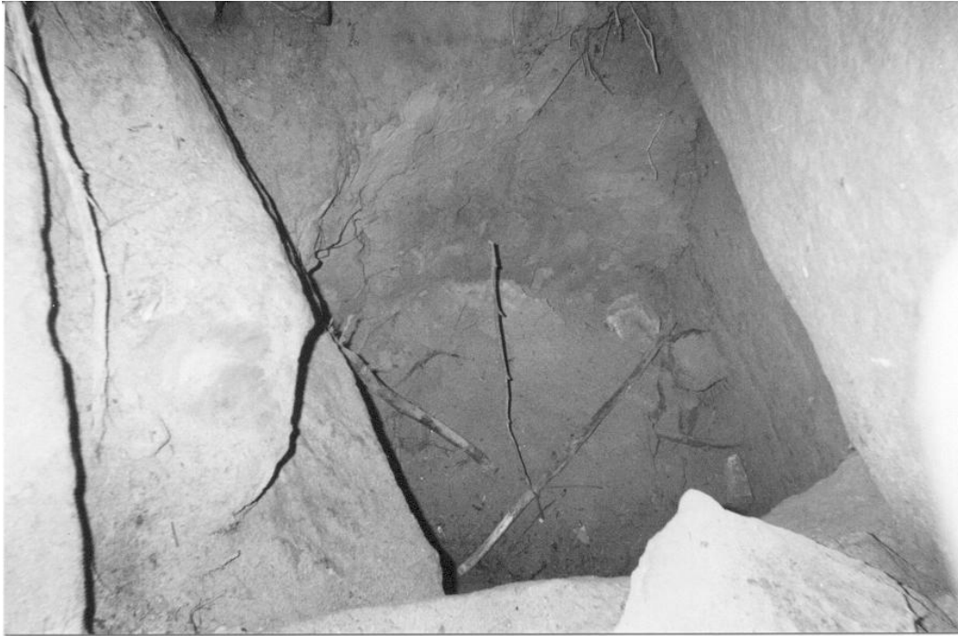
Section 3: The previous picture was taken from the bottom of this 80 by 80 centimetre excavation which, if the inscription of the pyramid hieroglyph is correct, should decent [down a stairway ?] into a lower chamber. © 2001 H-D von Senff
